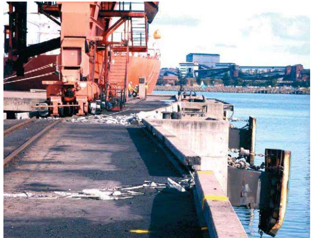
Damage to wharf (Australian Transport Safety Bureau, Marine Safety Investigation Report 178, 2002)
